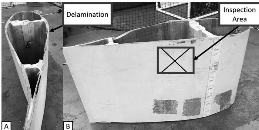
Figure 13.26: A – Wind turbine blade section end elevation view highlighting the internal delamination defect. B – Elevation view of the wind turbine blade section detailing the external inspection area.
